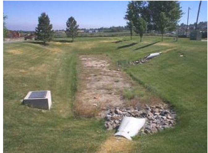
Sand Filter (no forebay) - Photo courtesy of Colorado UDFCD
